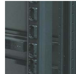
Embedded installation PDU
