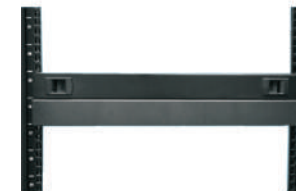
Blanking panel installation effect
