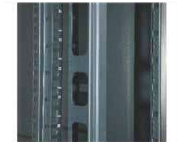
Metal cable management slot with cap
